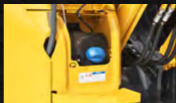
Ground level DEF tank
