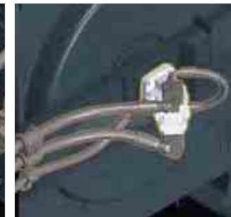
Hydraulic drive fan for oil cooler
